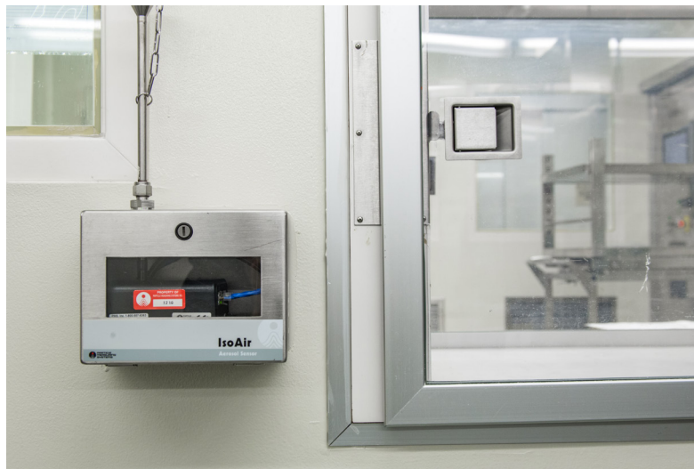
FIGURE 2 Airnet® II inside IsoAir® enclosure
